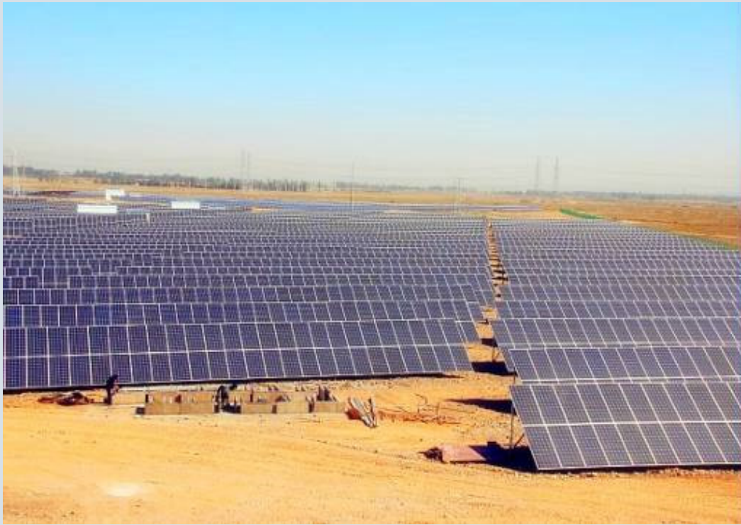
Jiuquan Dongdongtan 29MWp Solar Power Project
