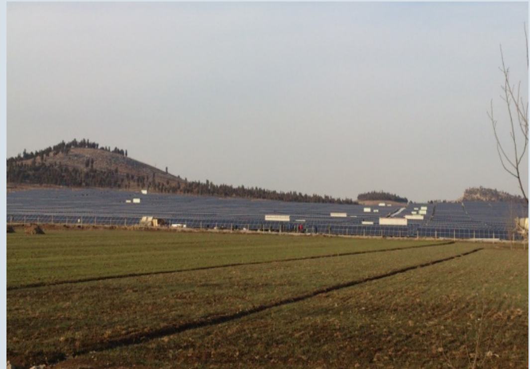
Jiangsu Pizhou 30MWp Solar Power Project
