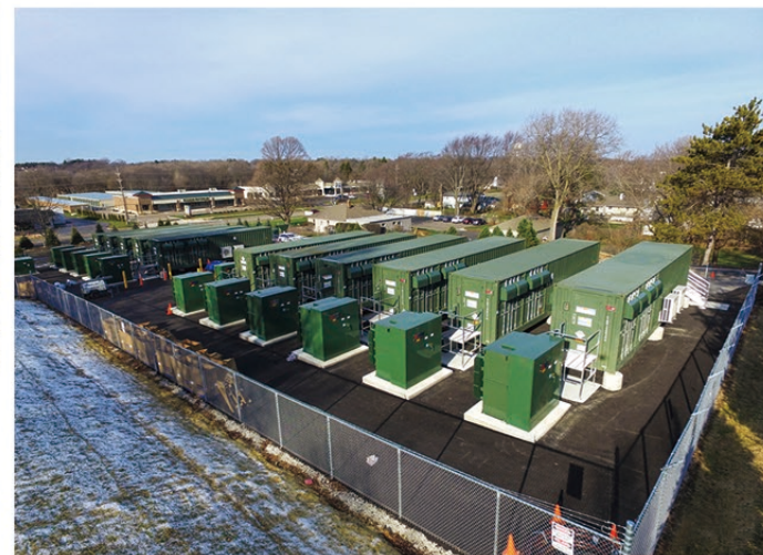
Chicago 19.8MW/7.865MWh ESS System Parameter Project Location: Chicago, USA Completion time: Jan. 2016 Owner: EDF Application: Frequency regulation
