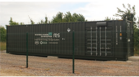
310 kW/668 kWh United Kingdom Completion time: Jun. 2016
