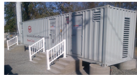
200kW/500kWh Charlotte, USA Completion time: August, 2012
