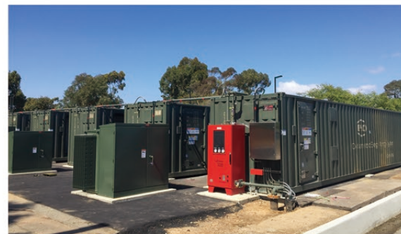
2MW/4.4MWh ESS Glacier, USA Completion time: Mar. 2016 Owner: PSE Application: Micro-grid
