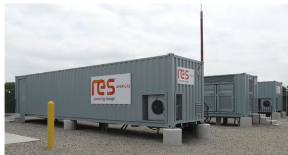
4MW/2MWh Ohio, USA Completion time: February. 2014 Owner: RES Application: Frequency regulation
