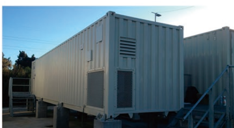
1MWh Sicily Italy Completion time: Mar. 2015
